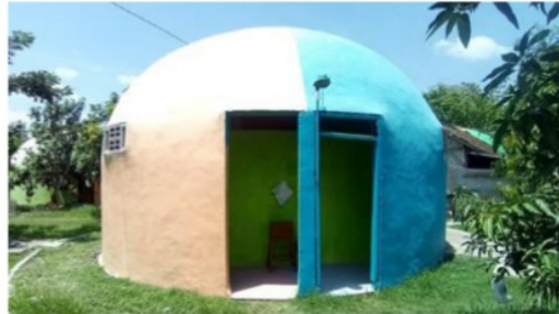
Communal toilets that are no longer functioning
