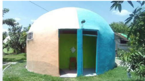
Communal toilets that are no longer functioning
