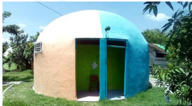
Communal toilets that are no longer functioning
