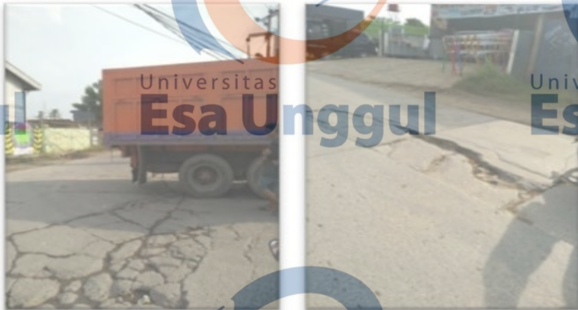
Picture 3. Condition of the Legok Street
