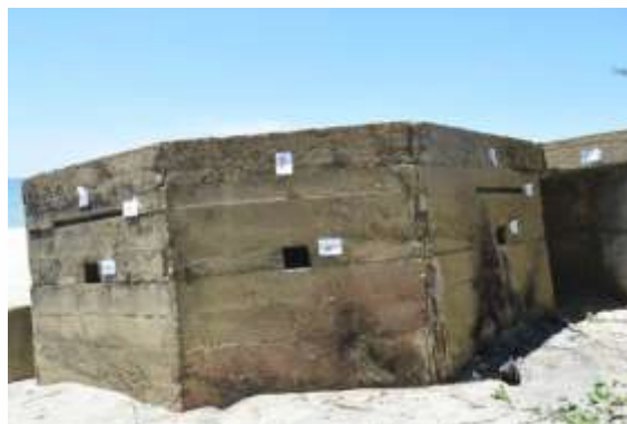
Figure 17: The structure of the British pillbox at Kg Pantai Chap, Bachok, Kelantan. Source: Field study.
