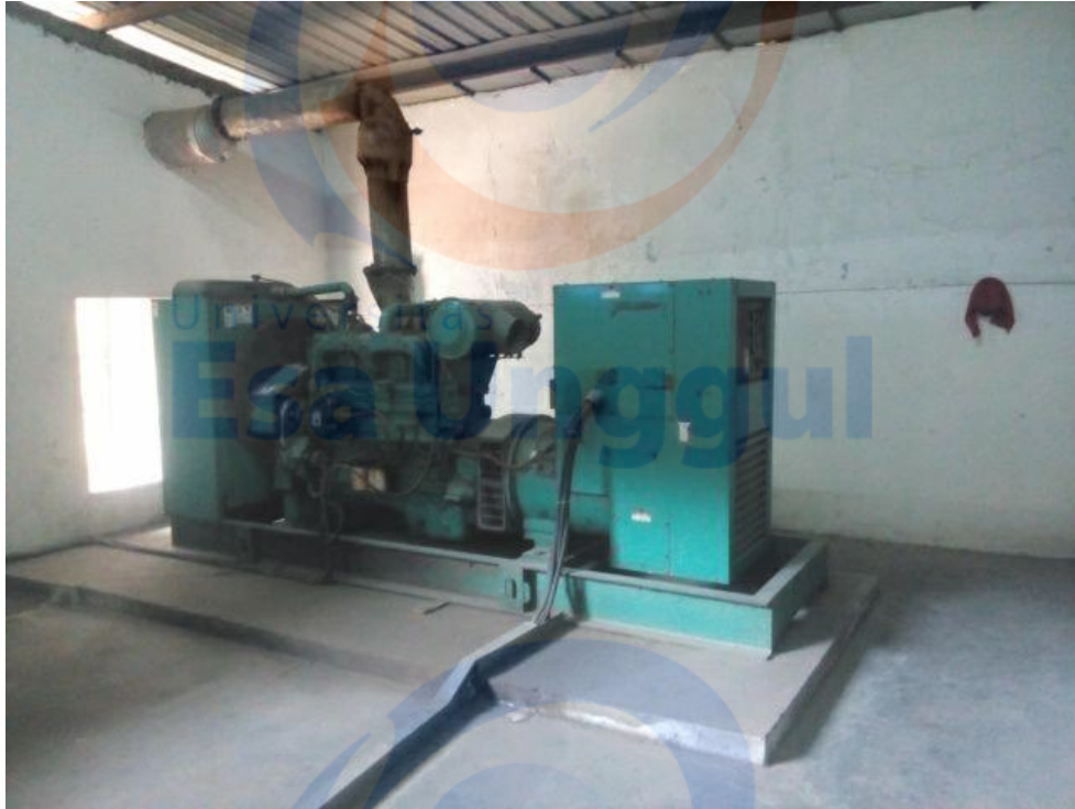
Genset PT SandangMutiaraCemerlang
