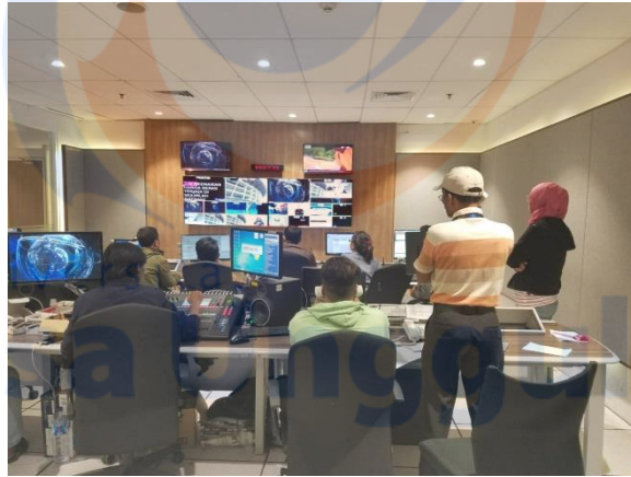
Ruangan Master Control Room (MCR)
